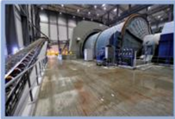
Milling, 2 parallel lines, each 25 MWe
